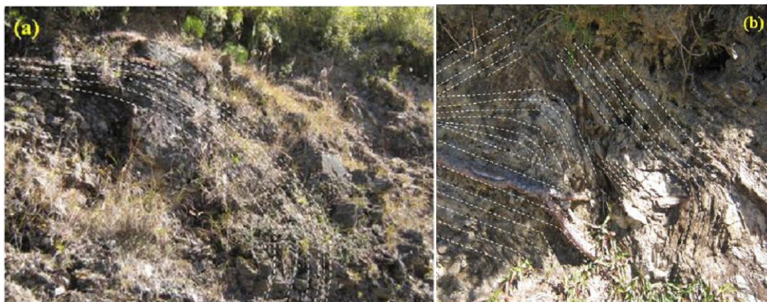
圖 2- 5 順向板岩邊坡拱彎變形露頭(Lo and Feng, 2014)
